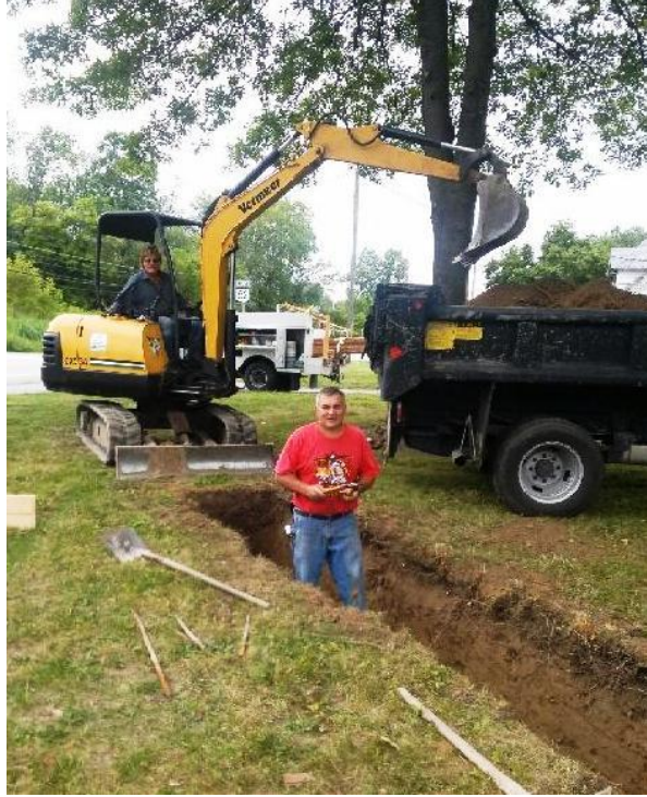
Wayne Brassell (left) and Ray Anthony work on preparing the footer for the new Columbia Clock Wall being constructed by the Columbia Community Foundation.
