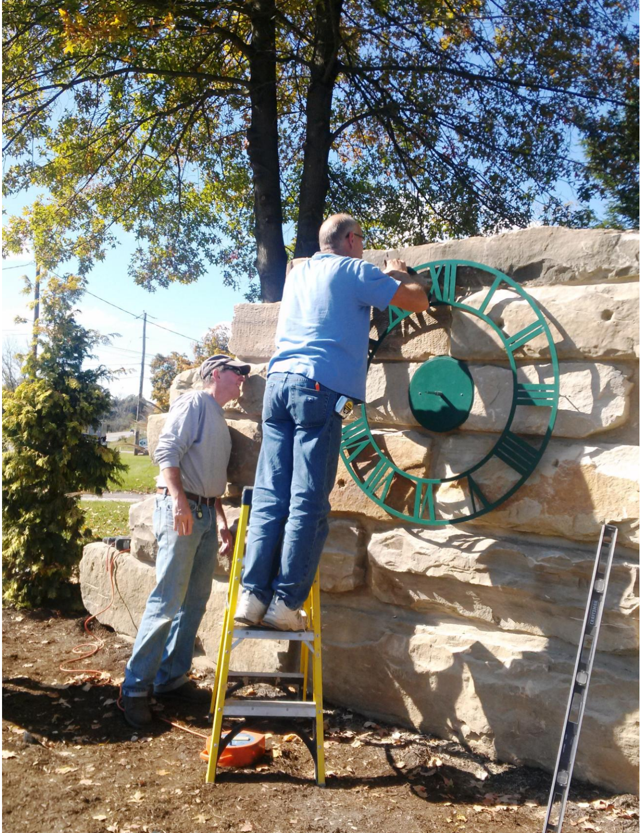
Crews work on installing the clock face on the Columbia Clock Wall project.
